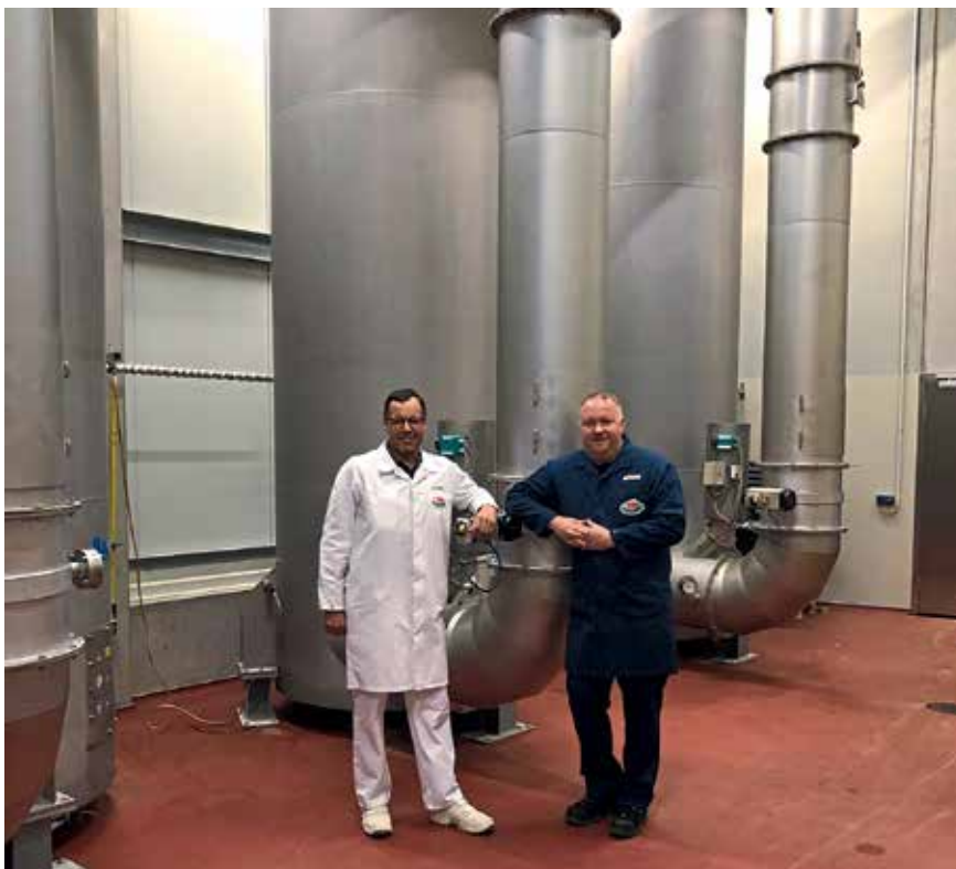
Division Manager Andreas Göhring (left) and Head of Industrial Engineering Bernd Goder are satisfied with the new smoke cleaning system.
